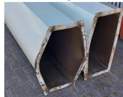
The damaged elevator casing
